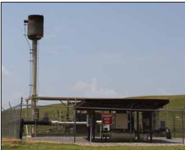
Methane Flare Station
